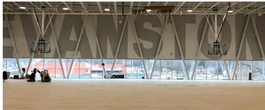
Top: A virtual mock up space of the gym at Robert Crown Community Center. Below: Robert Crown Community Center's gym under construction.
