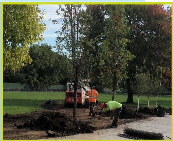
Workers install new trees at Lindberg Park as part of the 2014 renovation.
