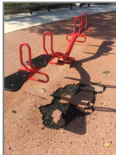
Poured in place surfaces at several playgrounds are starting to show wear. (Scoville Park)
