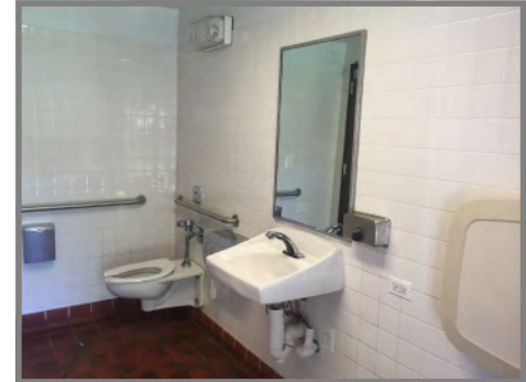
Overall, Park District bathrooms were in “Good” condition. Generally, bathrooms attached to community centers were in better condition than stand-alone facilities. For the 2nd year in a row, Andersen Park’s bathroom received a
