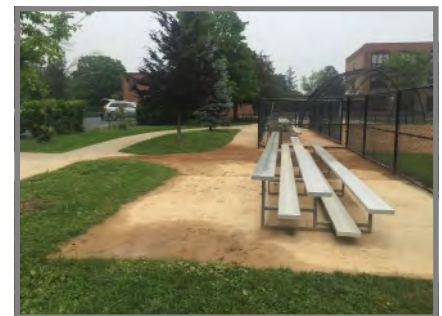
Despite turf and diamond surface improvements, other surface issues still exist, including migrating infield materials and deteriorating court surfaces. (Field Park)
