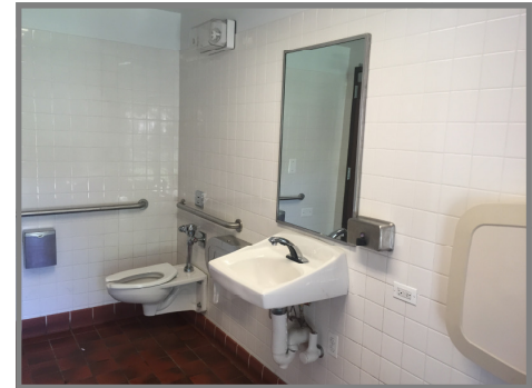
Overall, Park District bathrooms were in “Good” condition. Generally, bathrooms attached to community centers were in better condition than stand-alone facilities. For the 2nd year in a row, Andersen Park’s bathroom received a perfect score.
