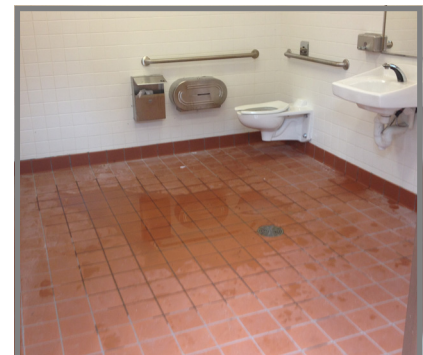
Some minor plumbing issues were found, including leaky sinks. (Scoville Park)
