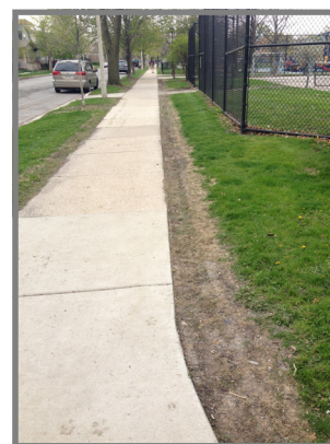
At many parks, the turf immediately next to the sidewalks was damaged from the winter snow removal process. (Longfellow Park)
