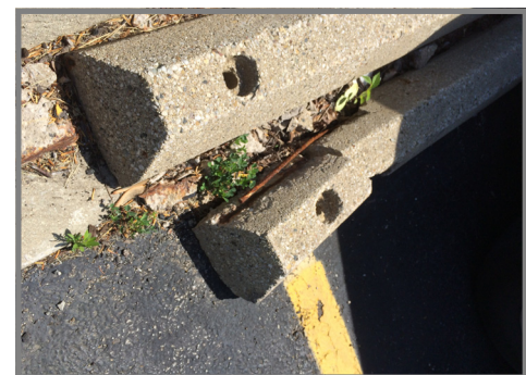
Bumpers were often broken and were missing from many parking spots. (Rehm Park)
