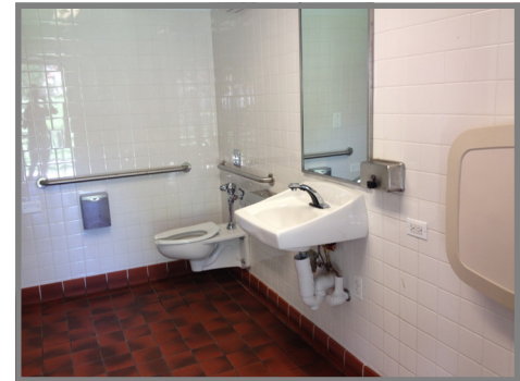
Overall, Park District walkways were in “Fair” condition. Generally, bathrooms attached to community centers were in better condition than stand-alone facilities. (Andersen Park)
